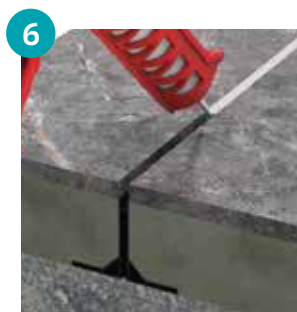
6 Joints are filled with suitable joint sealant or standard wedge joint profile
